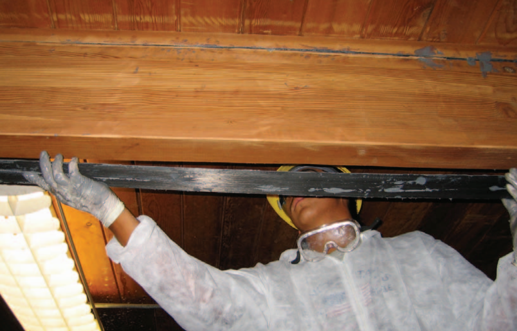
Figure 4: Installation of carbon plat near the top and on the tension faces of the beam
