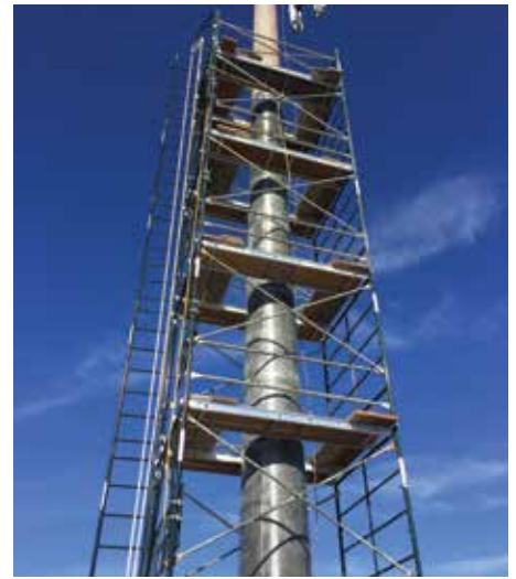
Figure 3. Carbon and glass FRP fabric applied to the lower 35 feet of the pole.
