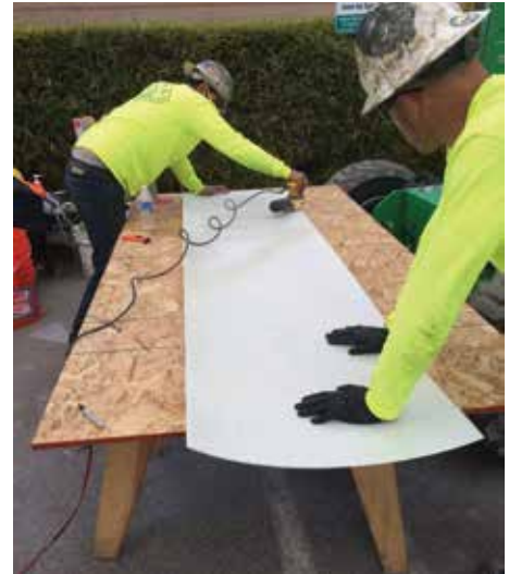
Figure 4. PileMedic laminates being cut to size on the job site before it is wrapped around the pole.
