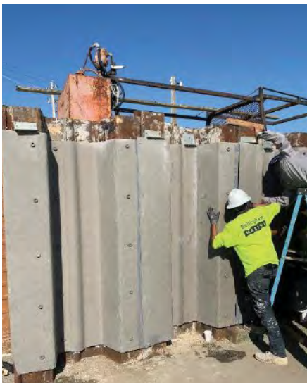
Bair Mock 5: Fit up of third and final panel for mockup. Photo courtesy QuakeWrap Inc.
