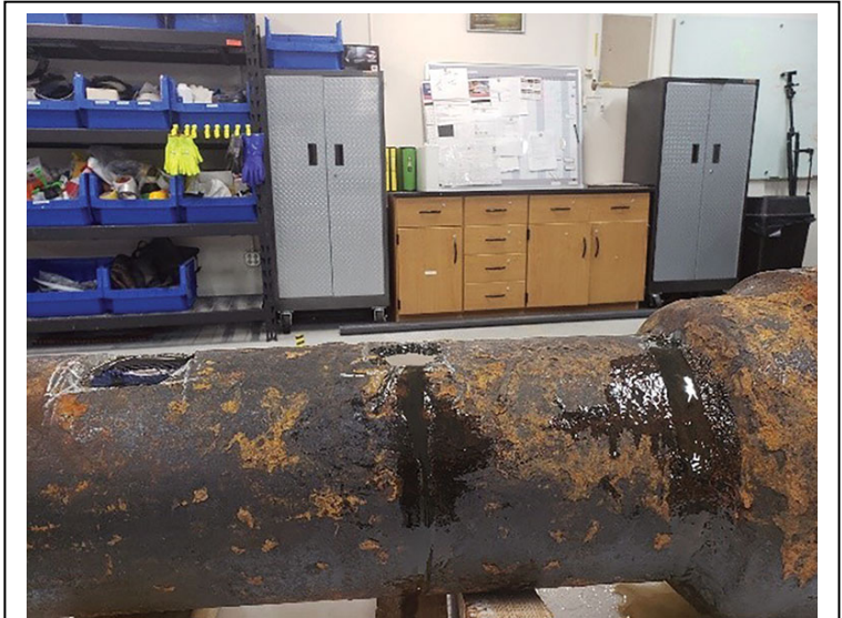
Figure 3: An unearthened cast-iron pipe repaired with SuperLaminate™ in the QuakeWrap Research and Development (R&D) Lab. Note the excess resin filling the holes cored on the pipe. (Photo: QuakeWrap)
