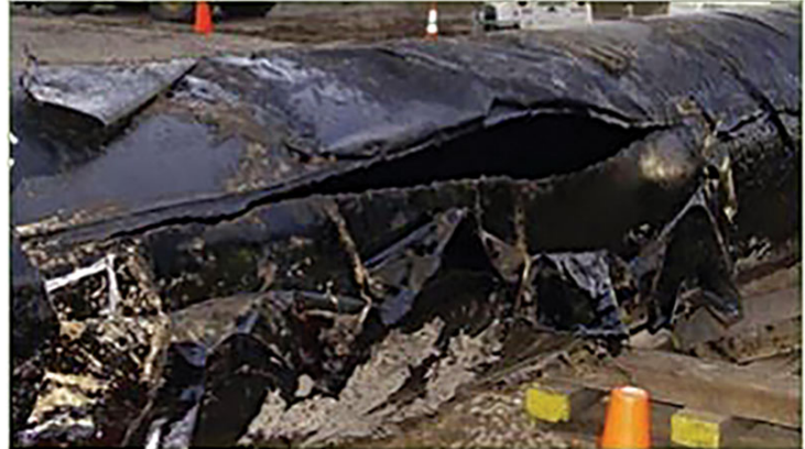
Figure 2: A steel transmission line failure due to corrosion and internal pressure.
