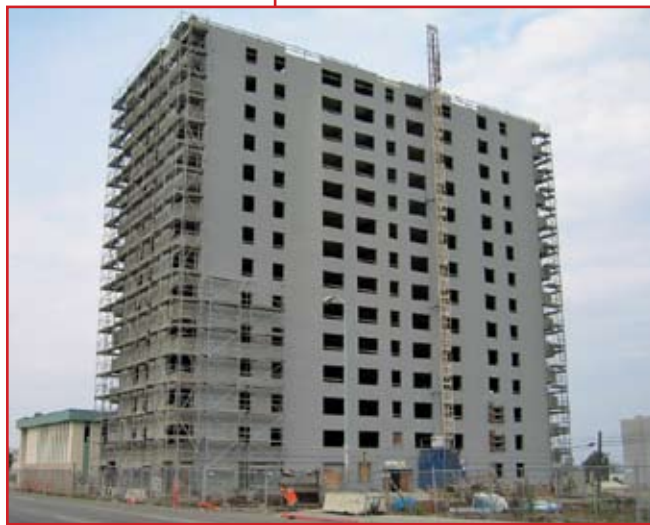
Figure 1: Damaged McKinley Tower sat vacant for more than two decades.
