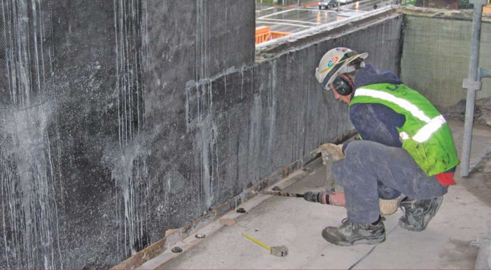
Figure 4: Retrofit of walls with carbon fabric and connection of wall to floor.
