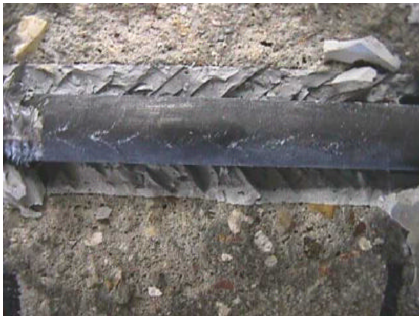
Figure 3.42. Internal Cracks in Specimen C3S6a
