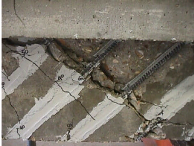
Figure 5.16. Failure of Beam B45-7
