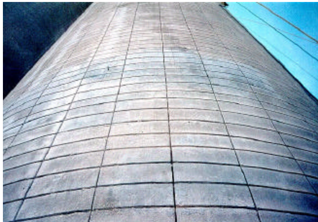
Figure 1.3. Grooves on the Surface of the Structure (Nanni, 1998)
