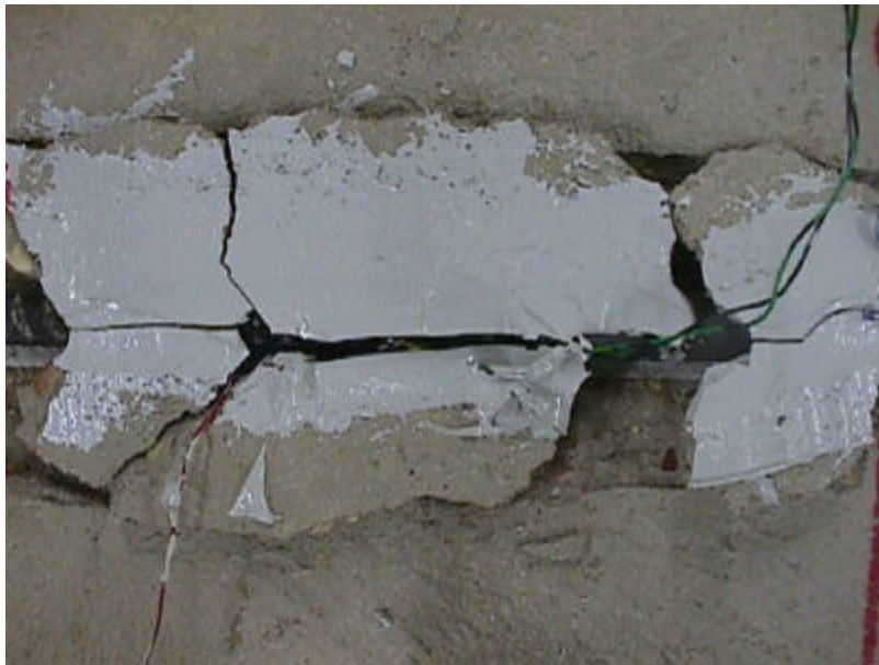
Figure 3.44. Crack Pattern in Specimen C3D24b After Failure
