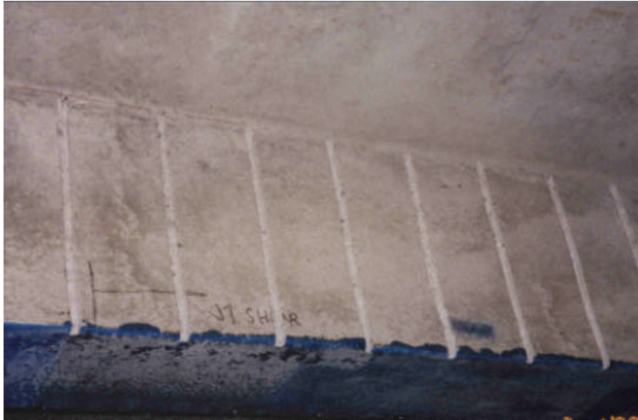
Figure 1.2. Vertical Grooves for Shear Strengthening with NSM FRP Rods (Hogue et al., 1999)
