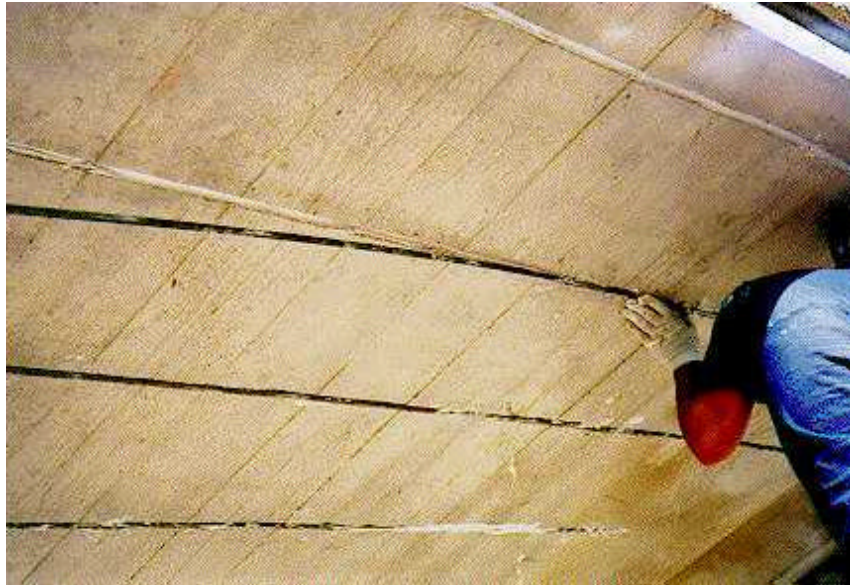
Figure 1.6. Installation of NSM CFRP Rods in the Bridge Deck (Alkhrdaji et al., 1999)
