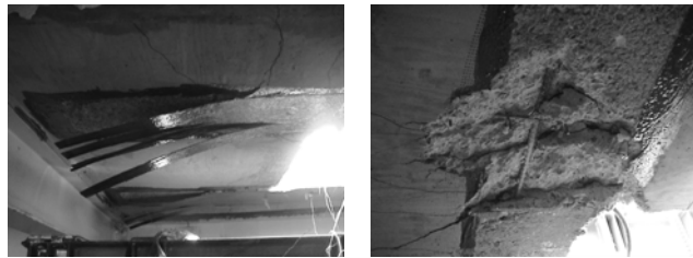
(a) Debonding of Laminates (b) Laminate-Concrete Bond
