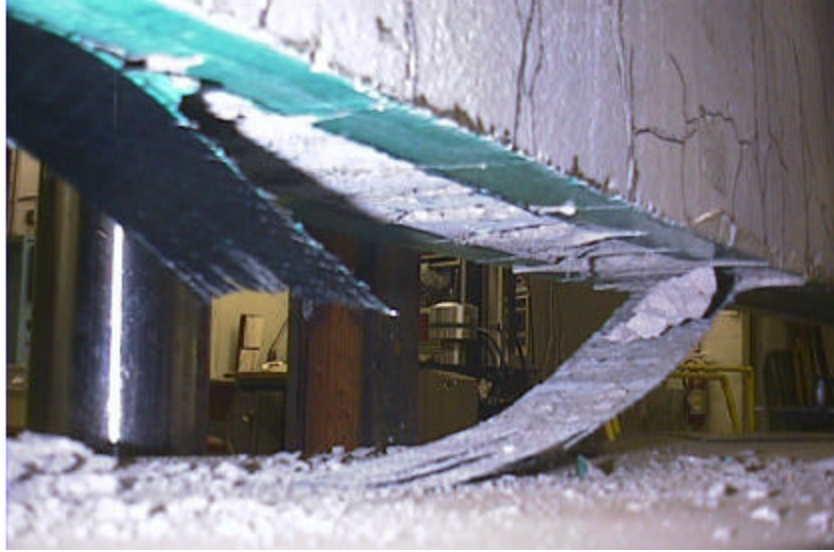
Figure 4.4. Final Failure in Beam A6
