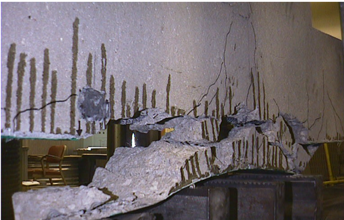
Figure B.2. Failure in Beam A1
