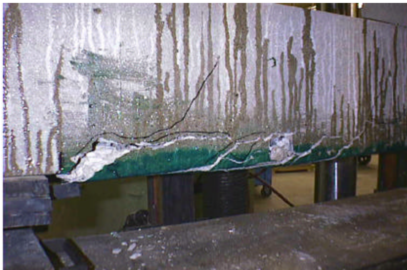
Figure 4.2. Final Failure in Beam A3
