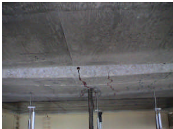
a) Flexural Failure (exposure of flexural reinforcement)
