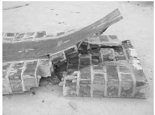
(f) Shear Failure (CL9)
