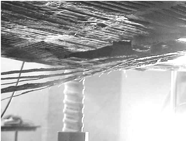
(a) Fiber Rupture (CL3)
