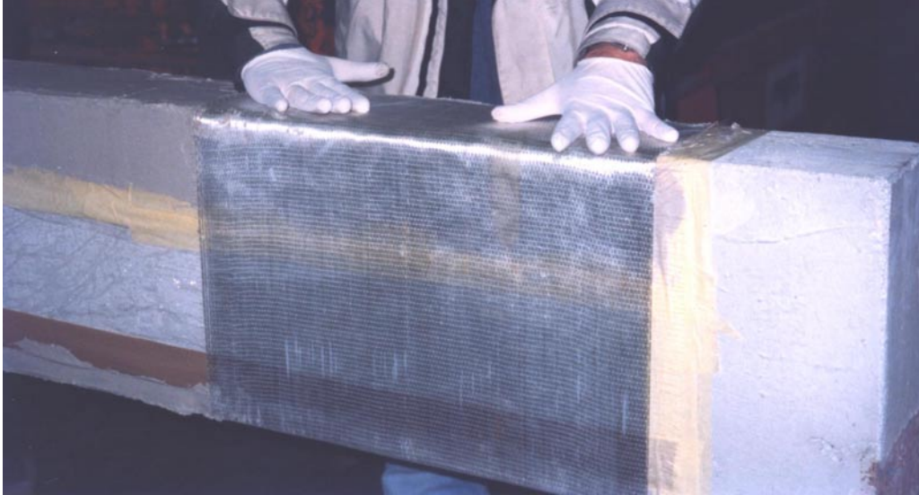
Figure 4: Beam ST1a: the preparation of the lateral surface and the application of the GFRP sheet
