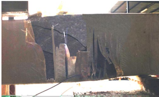
Figure 6: The beam ST1b at collapse
