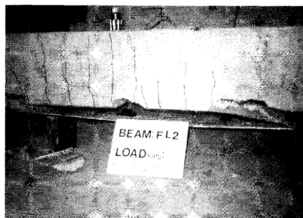
FIG. 2. Failure of Concrete Layer between FRP Plate and Tension Reinforcement
