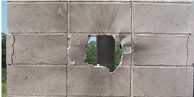
Figure 6.21 Front Side of Wall C2 after Event #1
