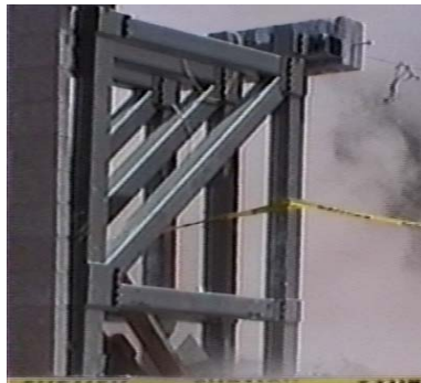
(c) Wall B1 Collapsed
