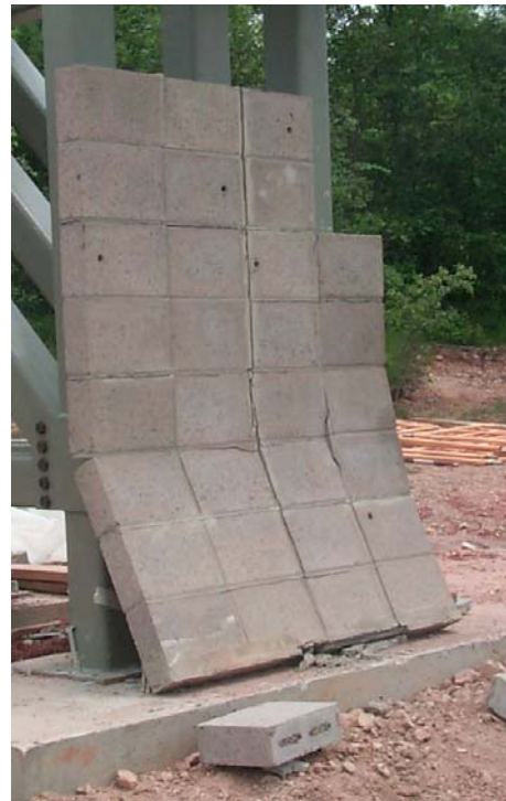
Figure 6.2 Failure of Wall U1 after Event #6
