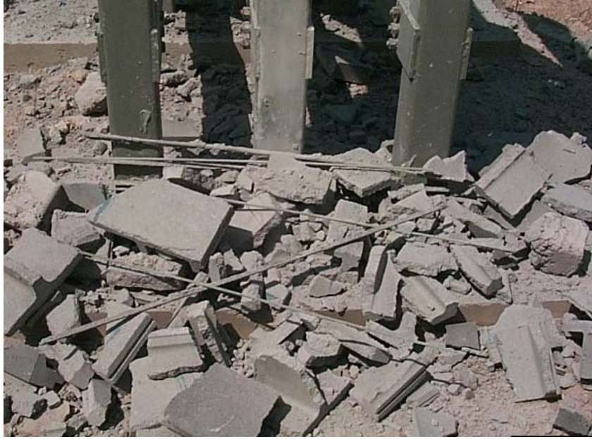
Figure 6.24 Total Collapse of Wall C2 after Event #3
