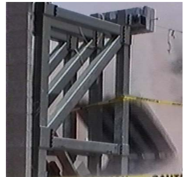
(b) Out-of-Plane Failure
