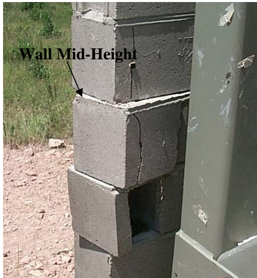
Figure 6.17 Wall A2 after Event #6
