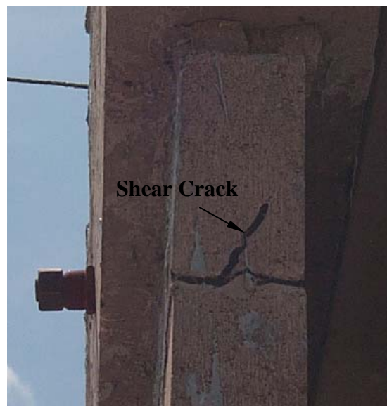
Figure 6.8 Shear Crack at Top Support of Wall C1 after Event #5
