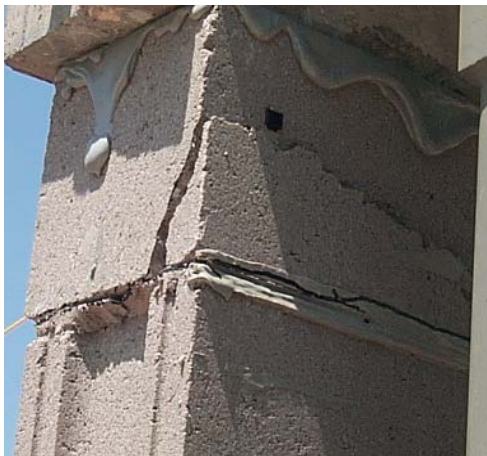
Figure 6.15 Shear Failure after Event #6
