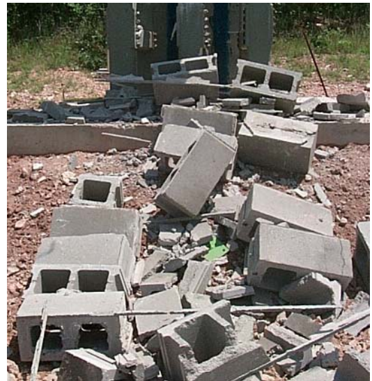
Figure 6.18 Collapse of A2 after Event #7
