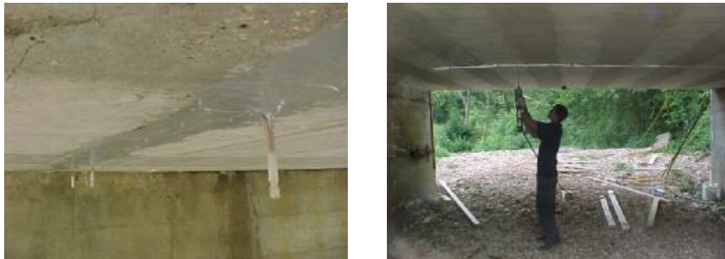
a) Crack Sealed Previous to Injection b) Crack Injection under the Bridge
