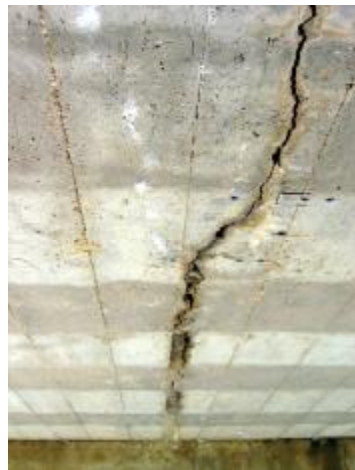
Figure 1-3 - Soffit Slab Longitudinal Crack
