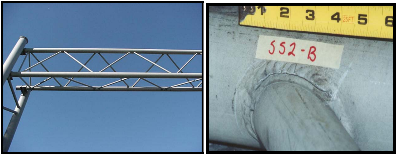
Fig. 1. Cracked welded connection: (a) overhead sign structure, (b) fatigue crack in welded connection of specimen SS2-B with a crack 66% of total weld length
