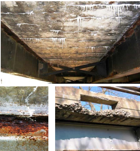
Figure 2 - Degradation of deck, girders and safety appurtenances of Bridge 1480230
